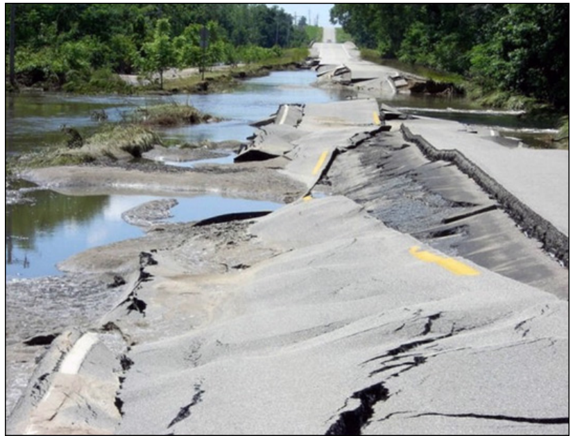
Damage to U.S. Highway 6 as the Cedar River subsides east of Atalissa in June 2008. Photo by Iowa Department of Transportation.
